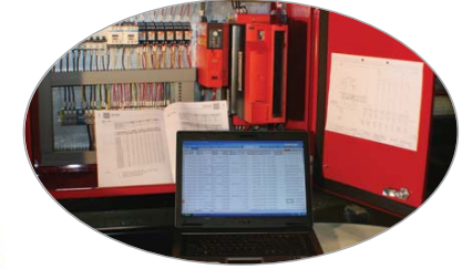
Elektrik Kontrol Paneli Electric Control Panel
