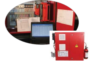
Elektrik Kontrol Paneli Electric Control Panel
